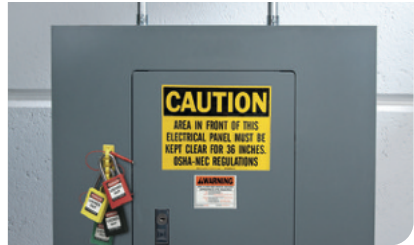
Panel and Enclosure ID
